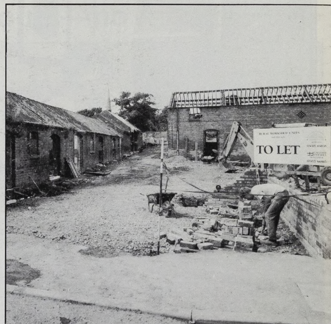
Jobs and conservation go together in this scheme in Ulceby, South Humberside where pig pens have become workshops.
