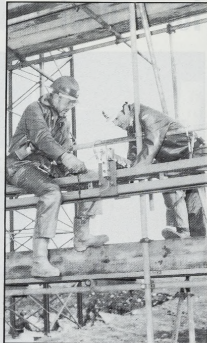
Fatal injuries to self-employed people in construction have nearly doubled in four years.
