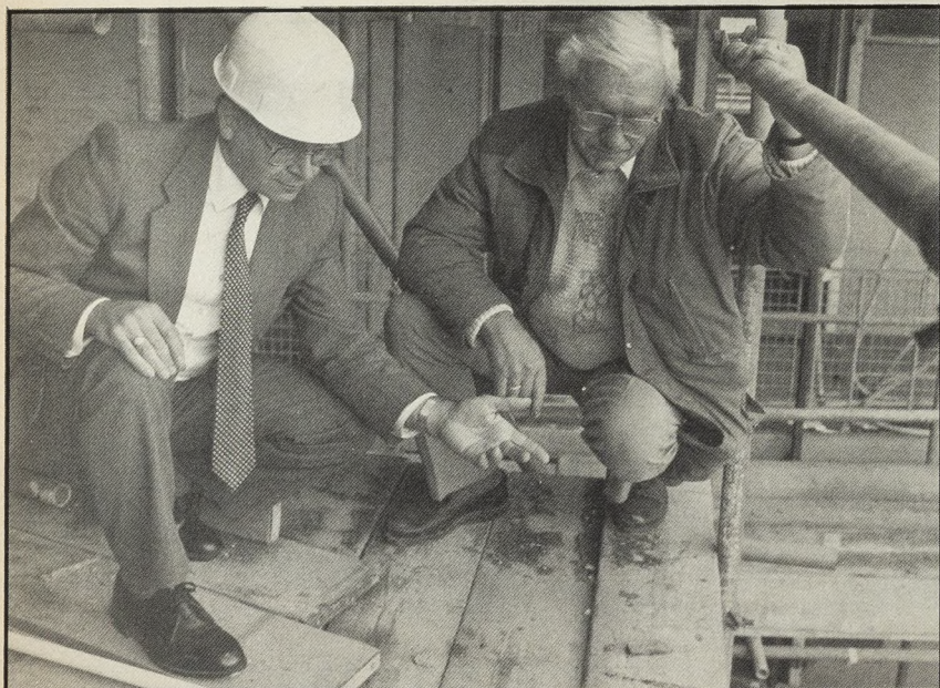
David Eves (left) points out a missing toe board to site agent, Reg Batson, during a "blitz" visit to a construction site in Camden, London.
