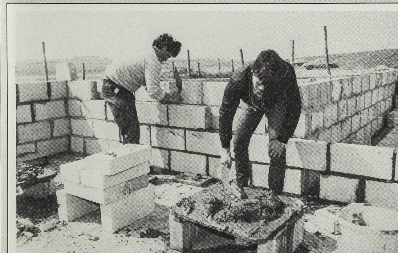
Building a shop and toilet block to open up a new stretch of tourist beach at Leysdon
