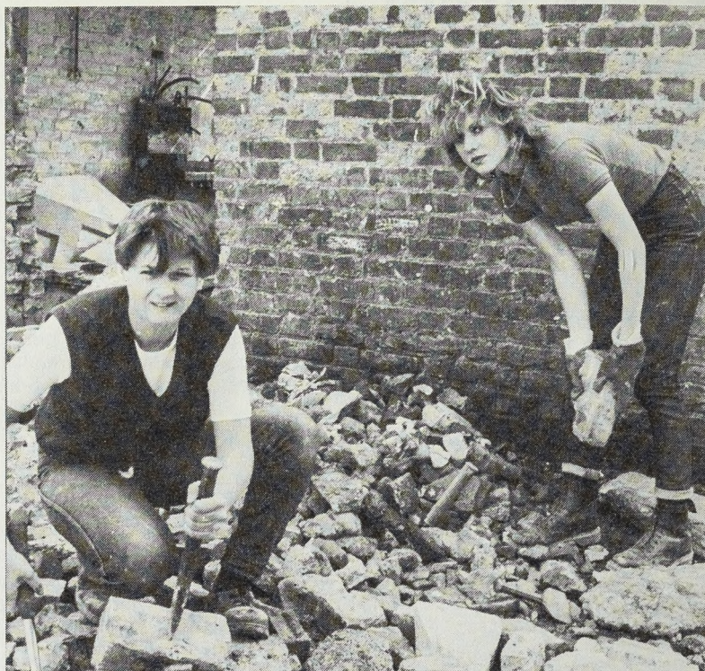
Laying the foundations for new skills: swim trainees try their hands at four different trades during their year in the scheme
