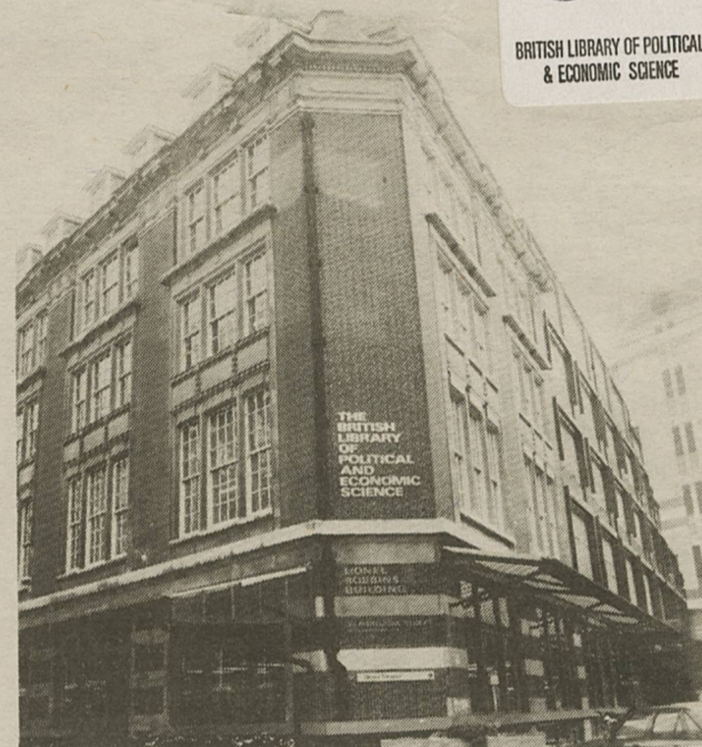
Consulting engineers have determined that the library's ceilings are in danger of collapsing. The ceilings' plaster finish is the biggest problem.
