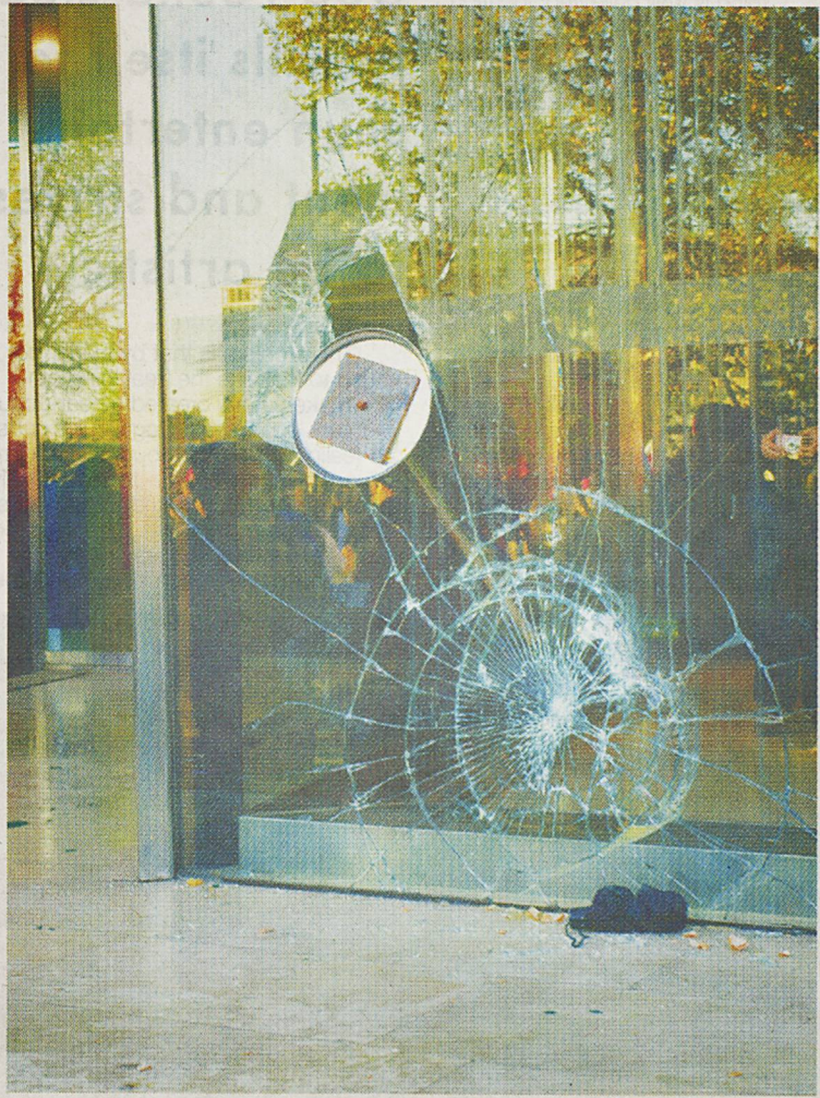
Disgrace: broken window!
