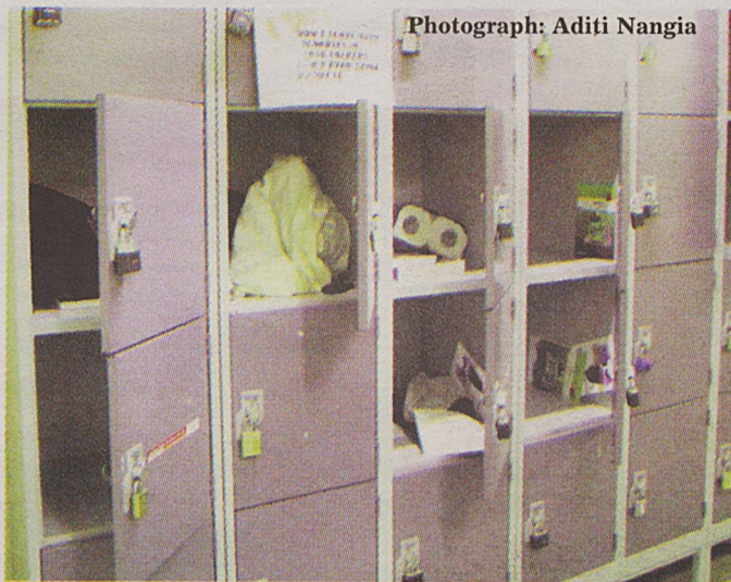
Photograph: Aditi Nangia A series of lockers broken into in the basement of the Old Building
